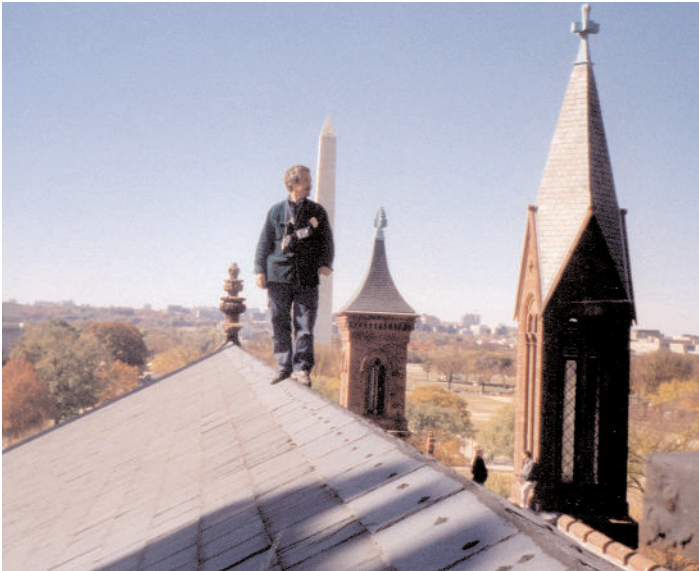
Figure 6: The Smithsonian Institution Building known as the Castle had already been replaced with new slate, but some of the original flashings had been left in place, and they leaked. The author is inspecting the roof in the photo above. Photographer unknown.
