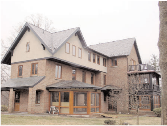
Figure 8: Ten year old slate roof on a private residence condemned by roofing contractors. The nominal snow guard damage, however, was covered by homeowner's insurance — the roof did not need to be replaced at all.
