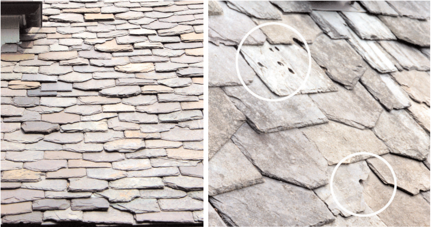
Figure 4: Chicago area home with beautiful 75 year old “ragged butt” slate roof condemned by three roofing contractors (above left). Hail damage as seen on Chicago area “ragged butt” slate roof (above right) is repairable by simply removing the damaged slates and replacing them. Most of the slates are undamaged. Photos by Joseph Jenkins
