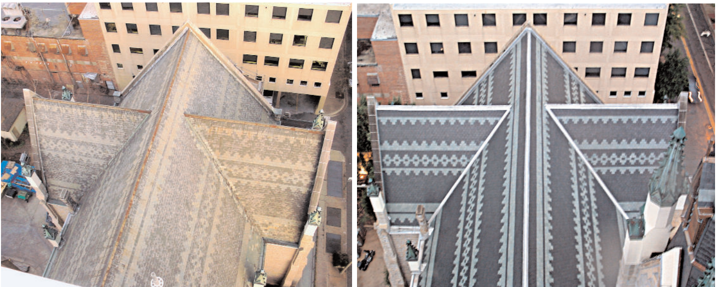
Figure 7: The Cathedral of St. Andrew in Little Rock, Arkansas, had worn out its black Pennsylvania slate after 120 years (above left). The Cathedral's new roof, installed by Midland Engineering in 2003, is likely to last 150 years. Vermont unfading green slate mixed with Welsh black slate and terne-coated stainless steel flashings should out-perform the original roof. Left photo by Joseph Jenkins; right photo by Lyle Bandurski.
