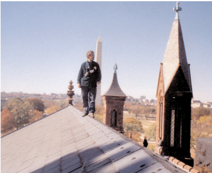
Figure 6: The Smithsonian Institution Building known as the Castle had already been replaced with new slate, but some of the original flashings had been left in place, and they leaked. The author is inspecting the roof in the photo above. Photographer unknown.
